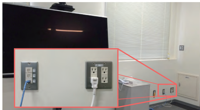
Figure. 4-1 network sockets (left), Power socket (right)
